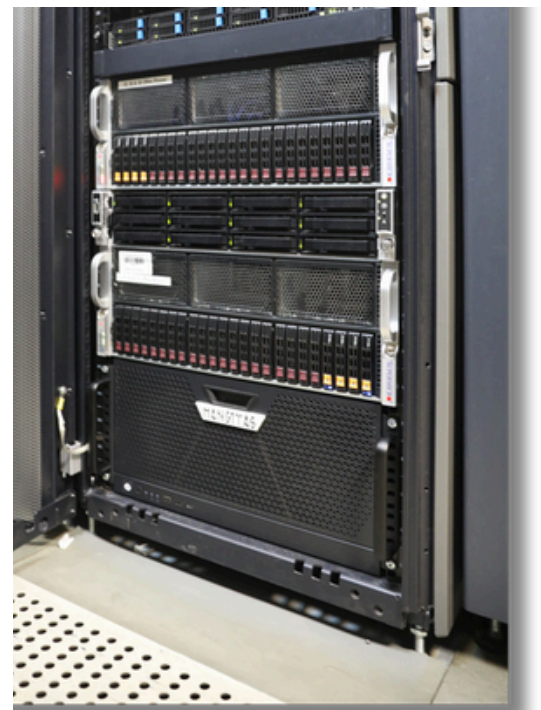
Nazarbayev University Data Center (Server room)
